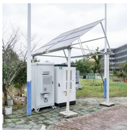
TCOM Solar Communication Tower
