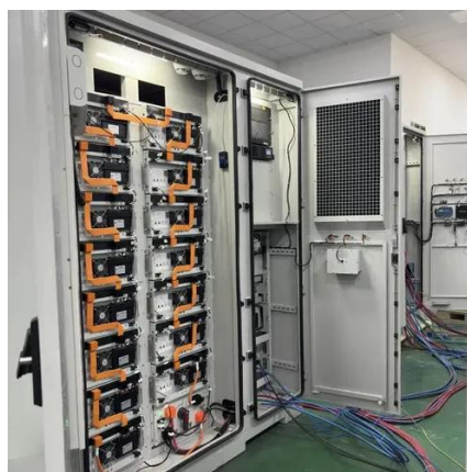
Hybrid Distributed Wind and Battery Energy Storage Systems
