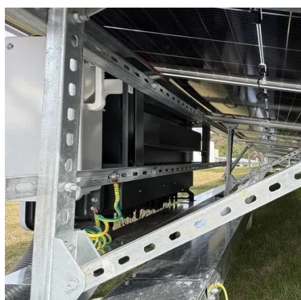
Wholesale bess storage system in algeria
