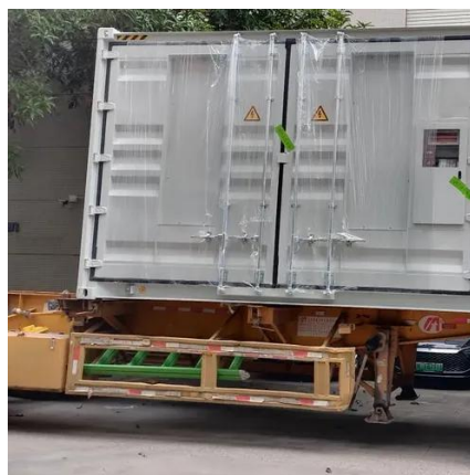
Floor-Standing Lithium Battery , SWA Energy LiFePO4 Storage
