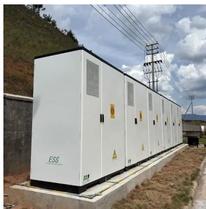
1.2MWh+600KW C& I BESS with Solar and Diesel Generator LiFePO4 Battery
