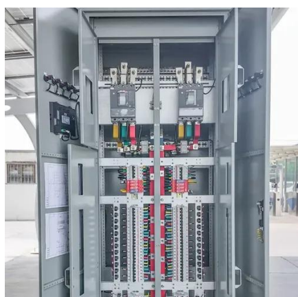
Perak power station
