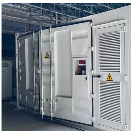
Outdoor Communication Cabinets and Power ...
