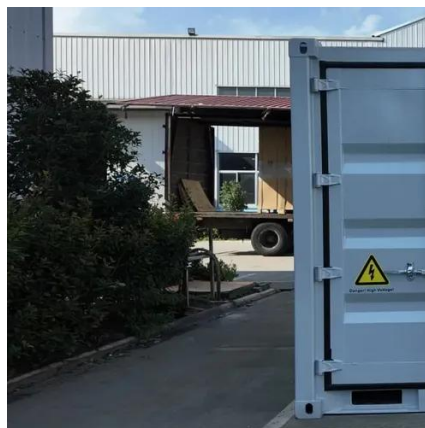
COMMUNICATION SITE ENERGY CABINET MANAGEMENT SYSTEM
