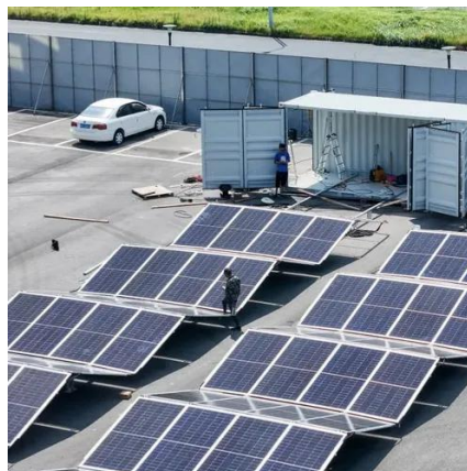
Senegal container energy storage cabinet equipment
