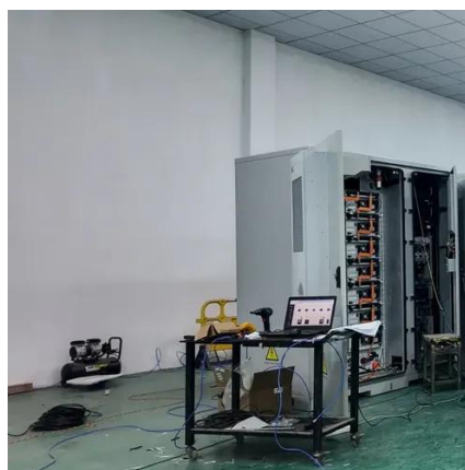
1MW Battery Energy Storage System
