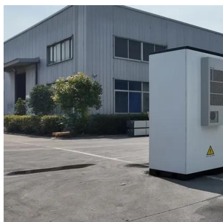
Telecom Equipment Cabinet
