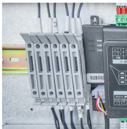
Industrial and Commercial All in One Cabinet-(100KWh+100KW)
