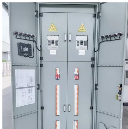
Oman power grid energy storage cabinet
