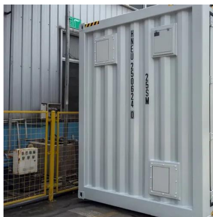
Flexible energy storage power station with dual functions of power ...
