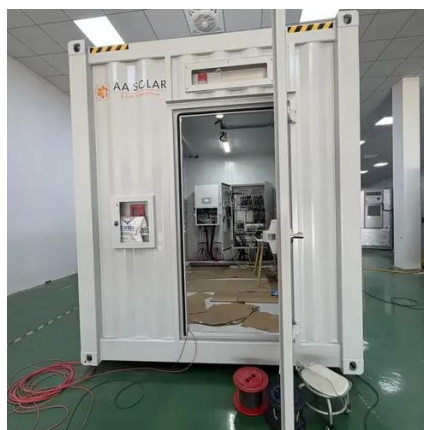
EnergyPack P200 , 188kVA 188kWh Battery ...
