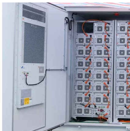
esm 48150a1 outdoor power cabinet
