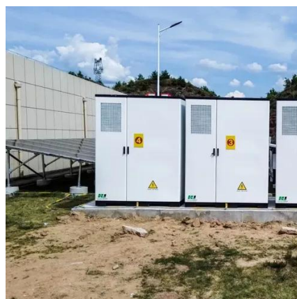
VRLA battery cabinets
