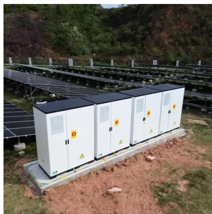
Liechtenstein Xitong BESS Power Station
