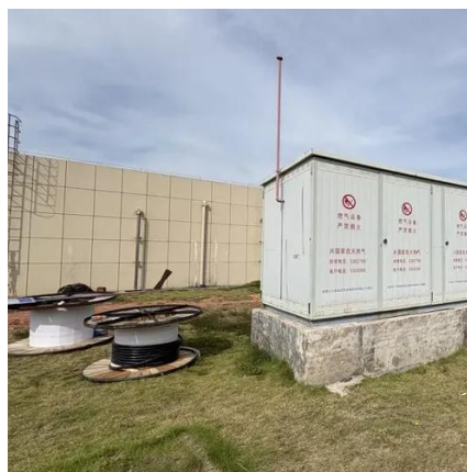
Photovoltaic energy storage cabinet battery point battery factory ...
