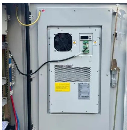
Photovoltaic Grid-Connected Cabinet , Low Voltage Distribution Cabinet
