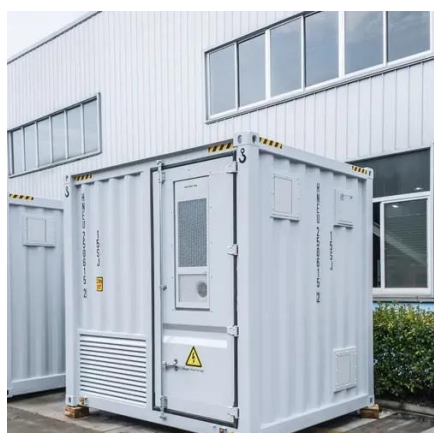
PHOTOVOLTAIC ENERGY STORAGE BATTERY CABINET
