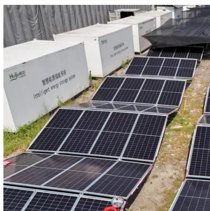
20-foot Air-cooled cabinet
