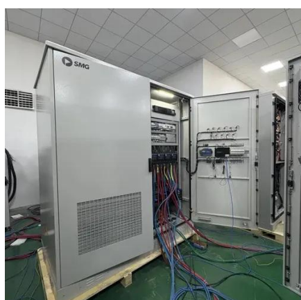
Addis Ababa EK outdoor power lithium battery
