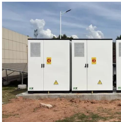
60KWh energy storage enclosure (external side mounted inverter)
