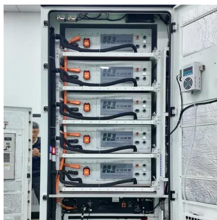
Outdoor Energy Storage System Cabinets , EPC Energy
