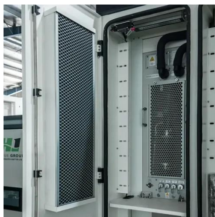
500kW/1075kWh Integrated Energy Storage System ...
