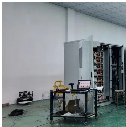
Energy storage container, BESS container
