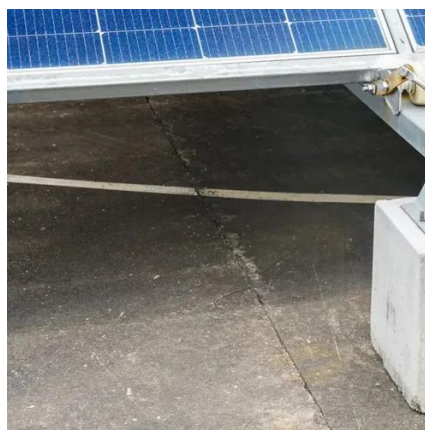
Outdoor cabinet C& I BESS
