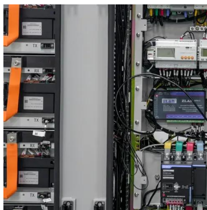
Commercial ESS 150kW/300kWh - EnSmart ...
